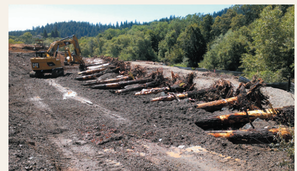
Huge root wads were used to provide bank stabilization and needed erosion control.
